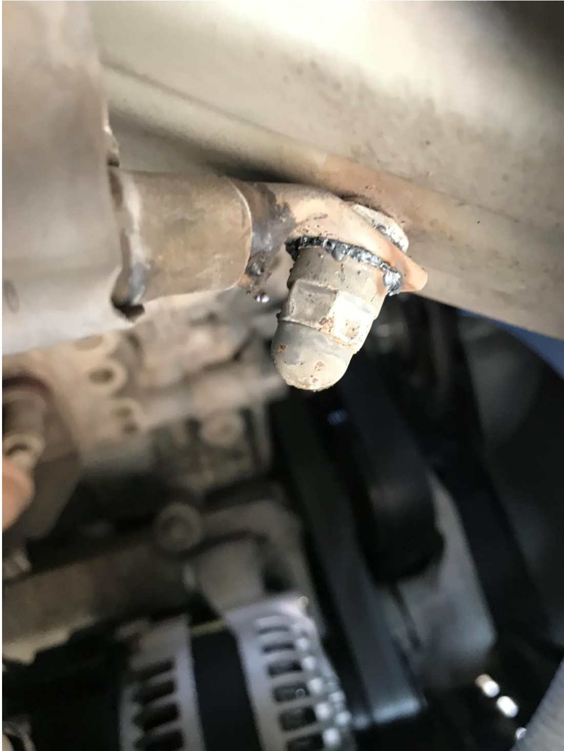
Close up of the battery ground cable, where it terminates on the body.
