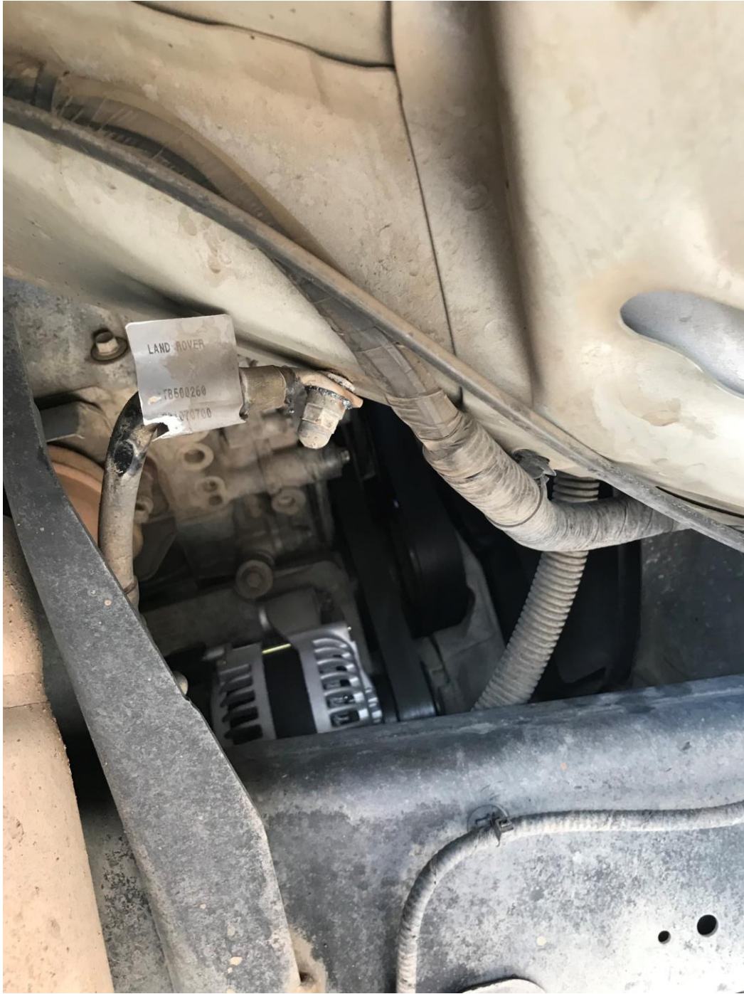
Inspecting the cable closely, you can see where it had been melting.
